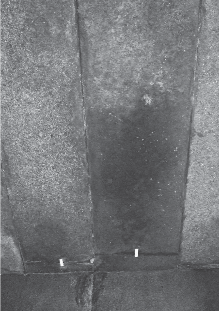
Plaster strips on the cracks in the King's Chamber help Egyptologists detect if the cracks get larger.
